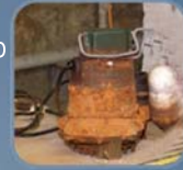
Sump Pump Failure
